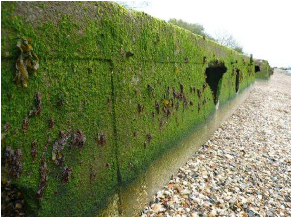
Figure 53 - Looking northwest up the line of Beetles - note the undamaged moss-free area at the base of the Beetles indicating beach motility and how the breaches in the side correspond to this level
