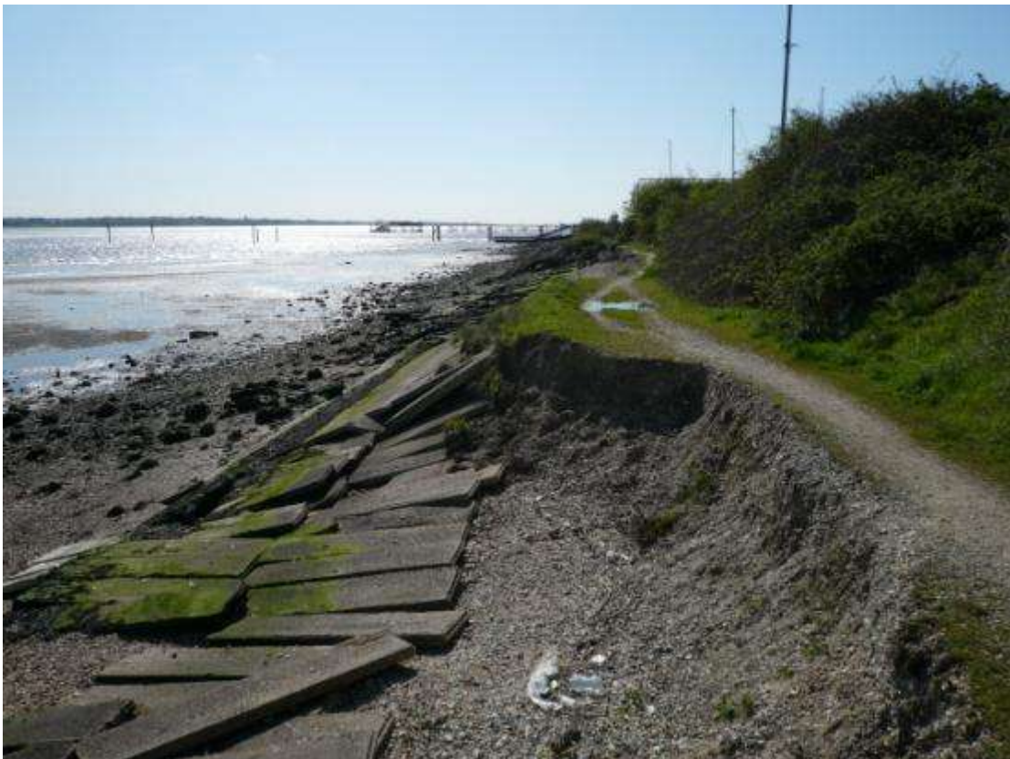
Figure 3 - Photo looking back towards Hythe from south of the site, showing local failure of the coastal defences
