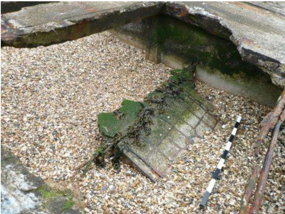
Figure 58 - Collapsed section of a Beetle, clearly showing the eroded metal reinforcements
